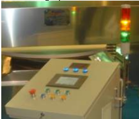
automatic and manual command buttons and lightened signal lamp.
